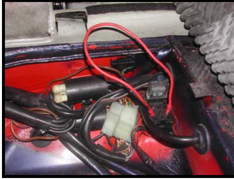
Picture showing Jumper Lead Installed
