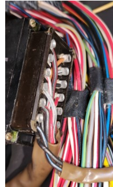
Cap removed from lamp controller plug
